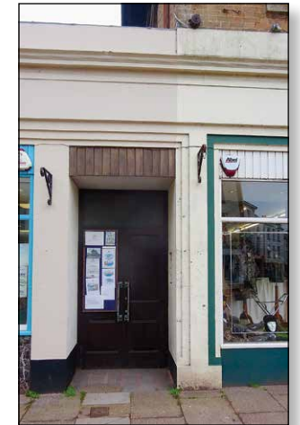
The entrance to the Town Hall needs upgrading.
