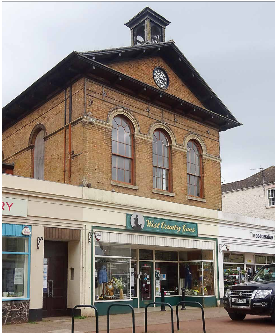
Town Hall from the Square; external repairs and redecoration are necessary.
