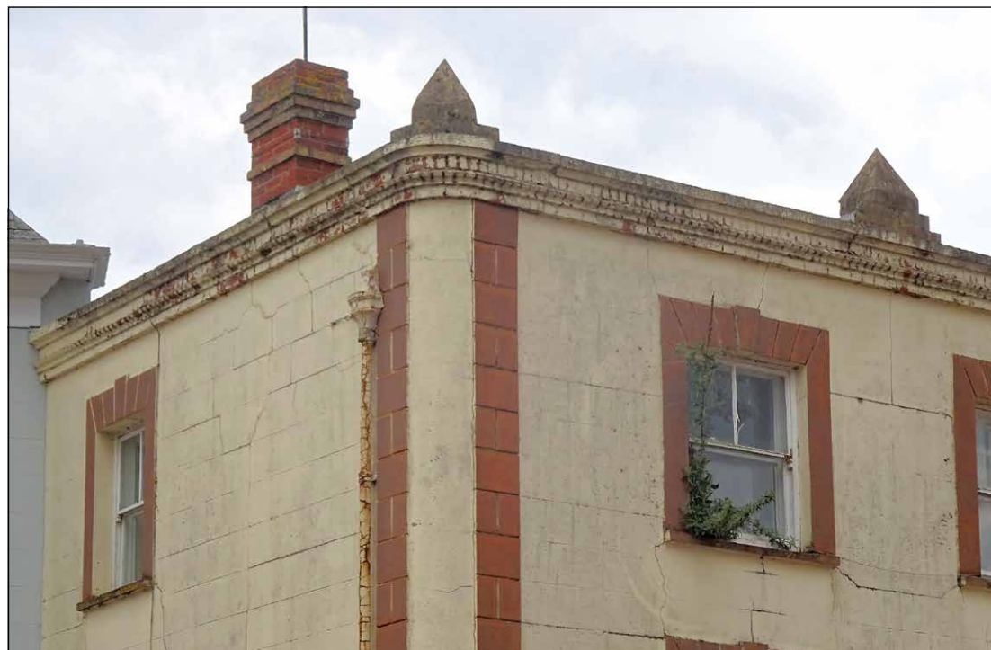
No.1, The Square – poor condition of upper floors.
