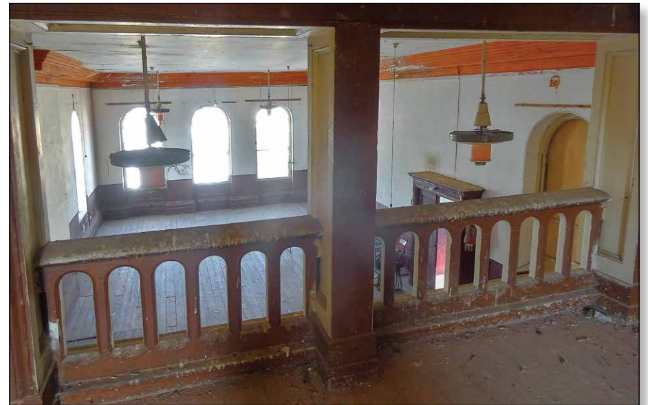
The interior, whilst generally intact, requires repair in places and redecoration.
